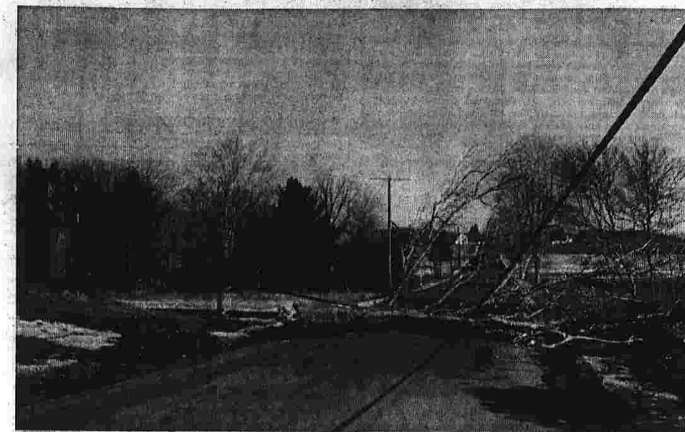
Strong winds this morning toppled this tree on Hilltown Rd. near Spencer St. It fell against a utility pole and snapped it, disrupting electrical power in the area. Power was off from 9:46 a.m. to 11:14 a.m., a Hartford Electric Light Co. spokesman said. (Herald photo by Saterini)
